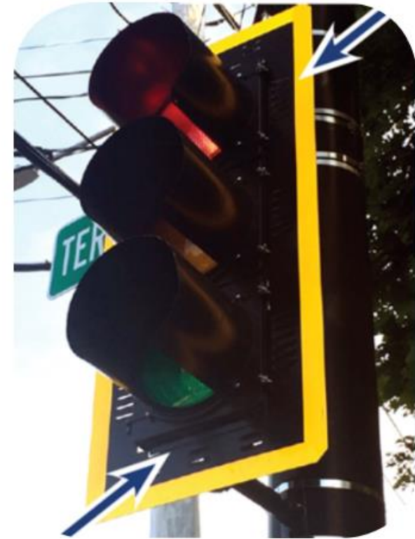
Retroreflective Backplates (FHWA)
